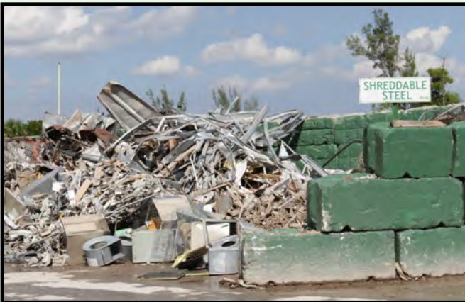
Steel, aluminum, brass and copper are among the metals commonly recycled from C&D
