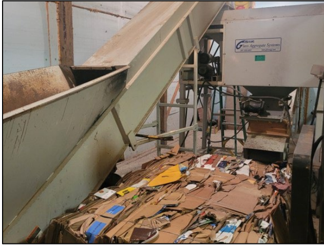
Figure 6: City of Tekamah glass grinder, showing hopper to pre-breaker
